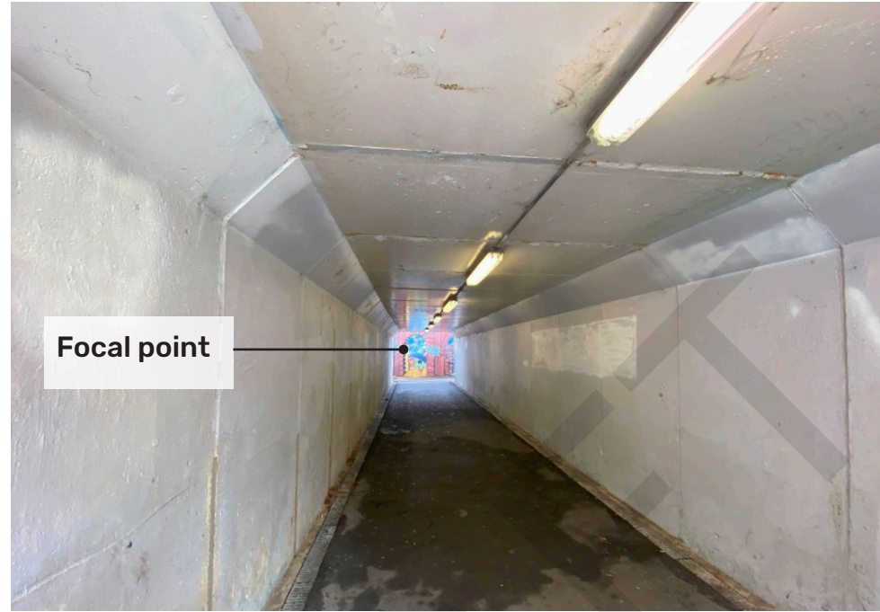
Tunnel is currently painted white which boosts lighting outputs. Any mural will naturally decrease light and needs to be capable of brightening the space. Mural at end is currently highlighting the destination. Maintaining this focal point should be considered in the tunnel mural design.
