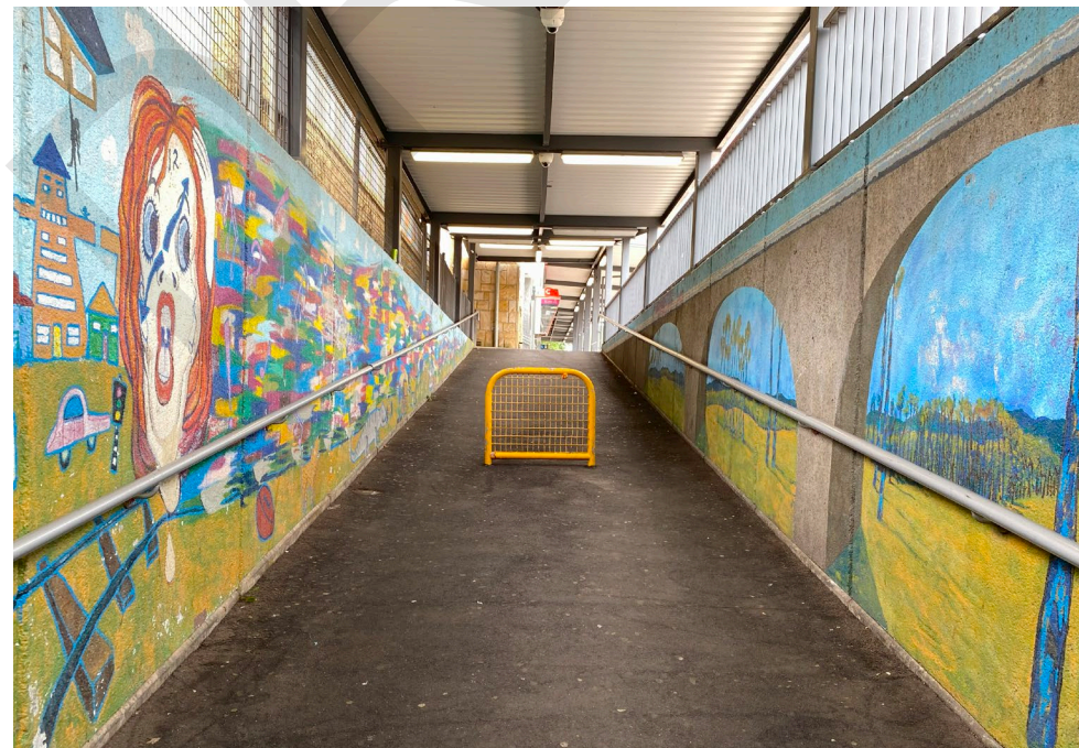
Ramp heading south to the entry to the station, on the western side of the rail line. Mural is on both sides of the ramp. The roof covering the ramp reduces light however, this side of the tunnel is brighter, likely due to the brighter coloured murals and lack of landscape between the footpath and the ramp.
