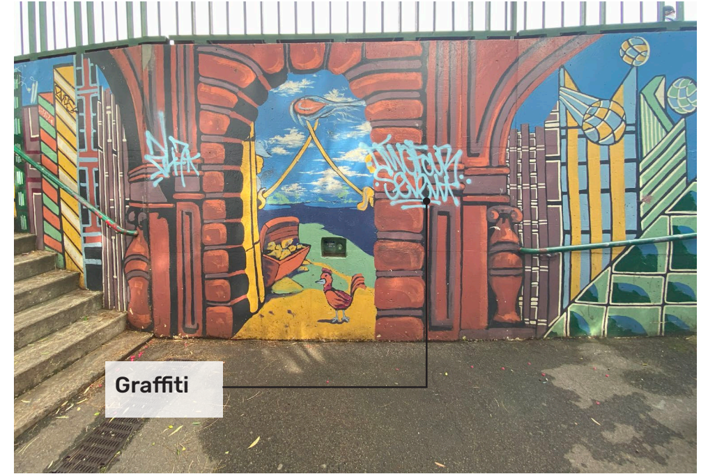
Artwork at the western end of the tunnel between stairs and ramp. Graffiti is observed on these murals.
