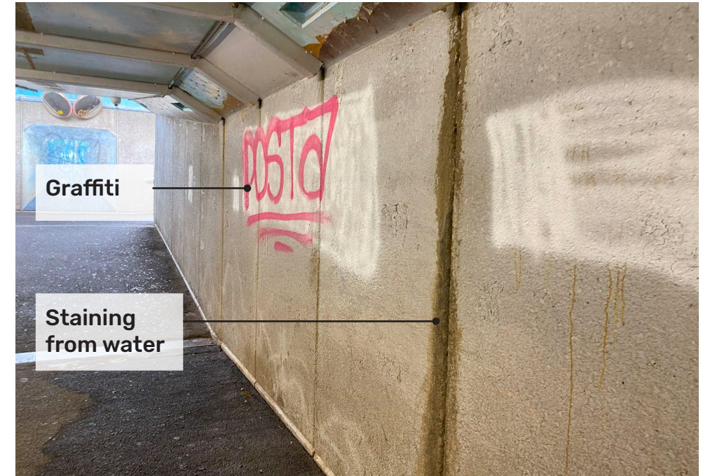
Graffiti painted over and then graffitied again. Staining is visible in this image. The water is not able to be stopped and the stain cannot be removed.
