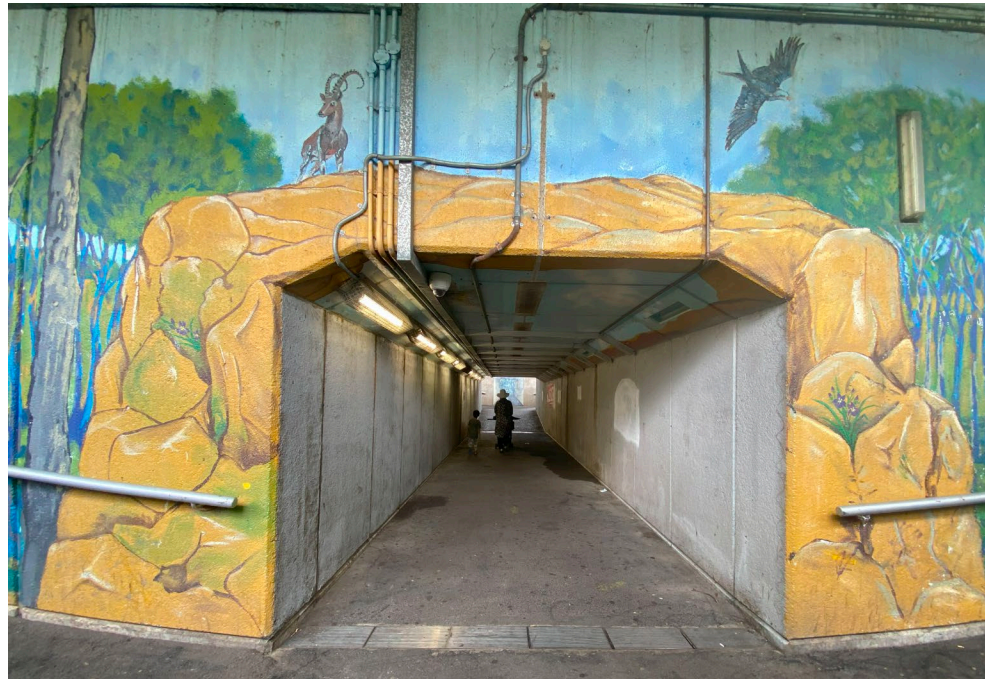
Tunnel looking west. Tunnel is XX long and previous murals, painted on panels have been removed and walls painted white. Roof retains former mural design. Lights have been relocated to the left corners. Some lights are not working resulting in gaps in lighting. Future creative lightning is strongly recommended.
