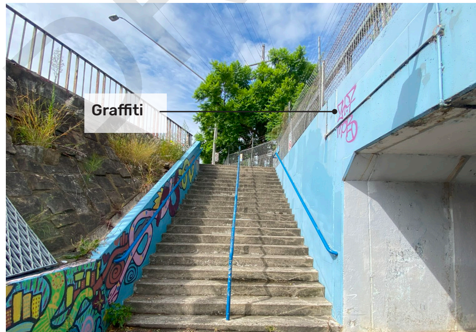
Looking up the stairs that connect to Railway Terrace. Weeds and grass grow in the retaining wall. Graffiti is observed above the tunnel.
