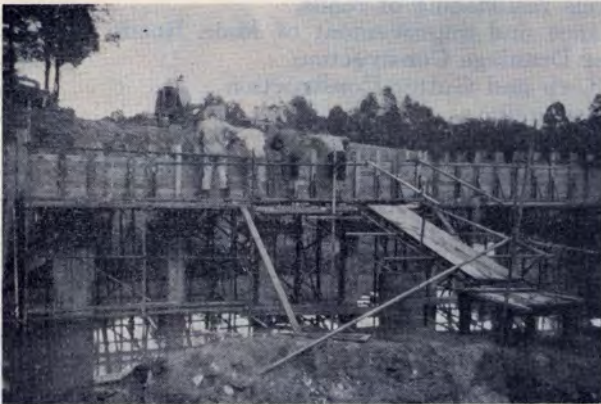
Here a modern pre-stressed concrete bridge replaces the plank of pioneering days.
